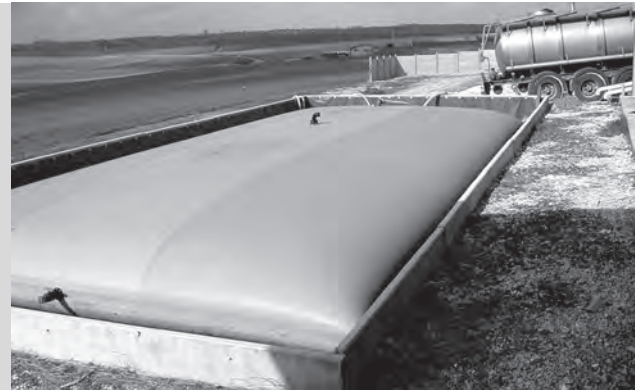
→ view of waterproof containment system for the tank
